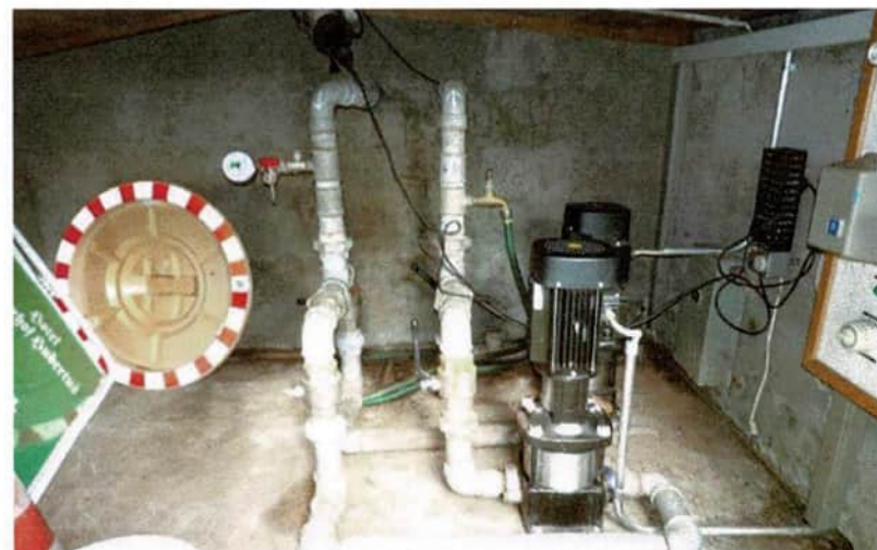
Installation Pumpenhaus Nr. 136B
